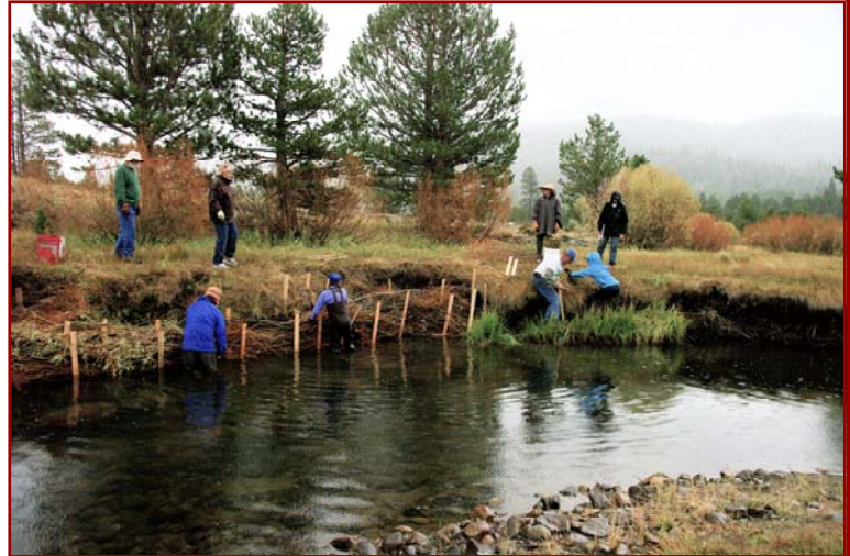
Volunteers stabilizing the river bank on the Carson River in Hope Valley.
