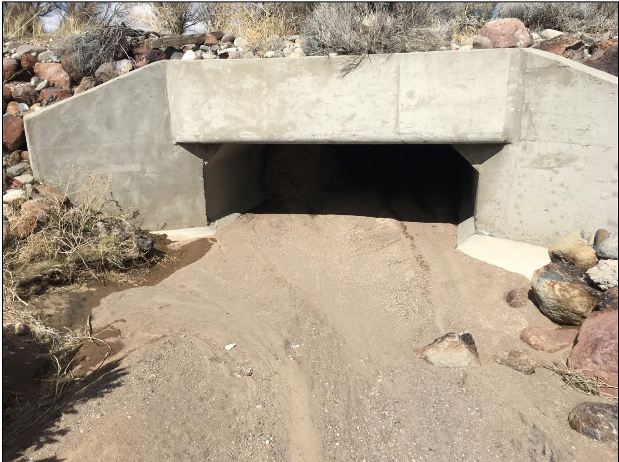
Figure 3-1. Example of sediment deposition at culvert
