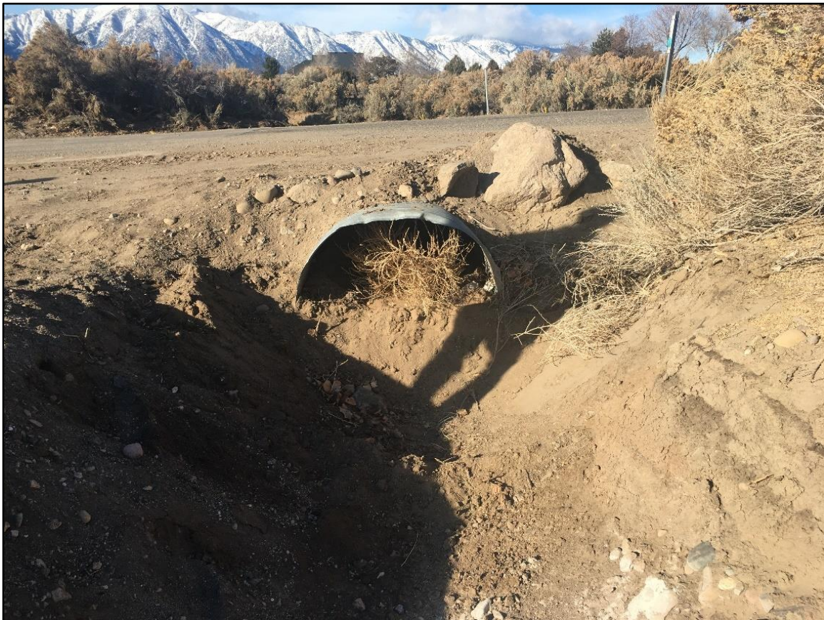
Figure 3-1. Example of sediment deposition at culvert
