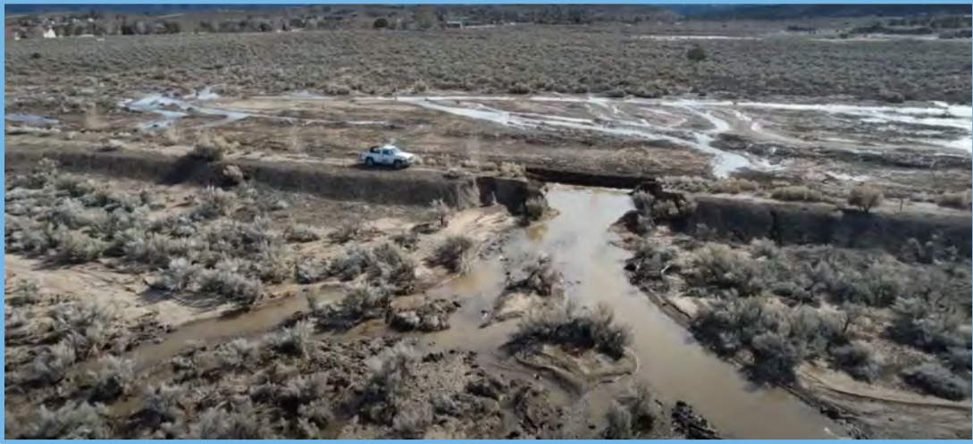
Figure 16: Damage to the Upper Allerman Canal in Douglas County in 2023 – Shane Fryer
