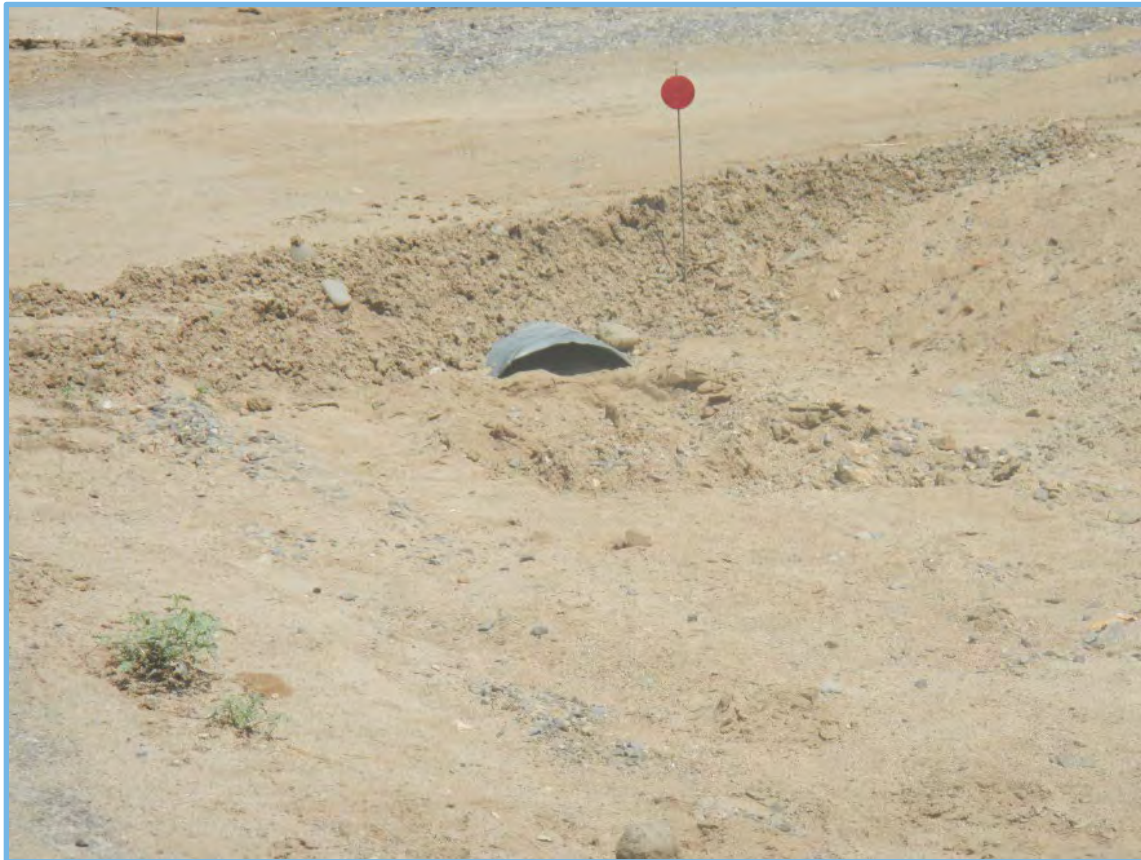
Figure 72: Culvert can quickly fill with mud and debris. Courtney Walker
